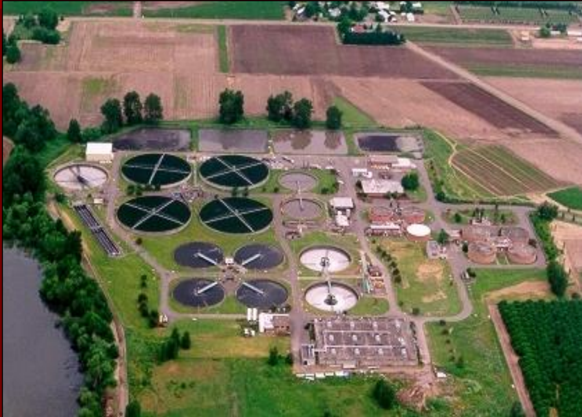
Wastewater treatment facility
